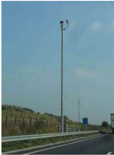
Figure 12 Typical mast mounted CCTV camera
