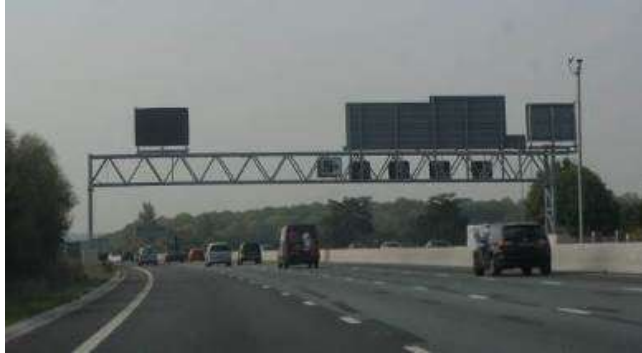
Figure 11 Typical super-span portal gantry
